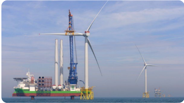
Wind Turbine Generators (WTGs)
