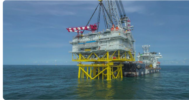
Electrical Service Platform (Offshore Substation)
